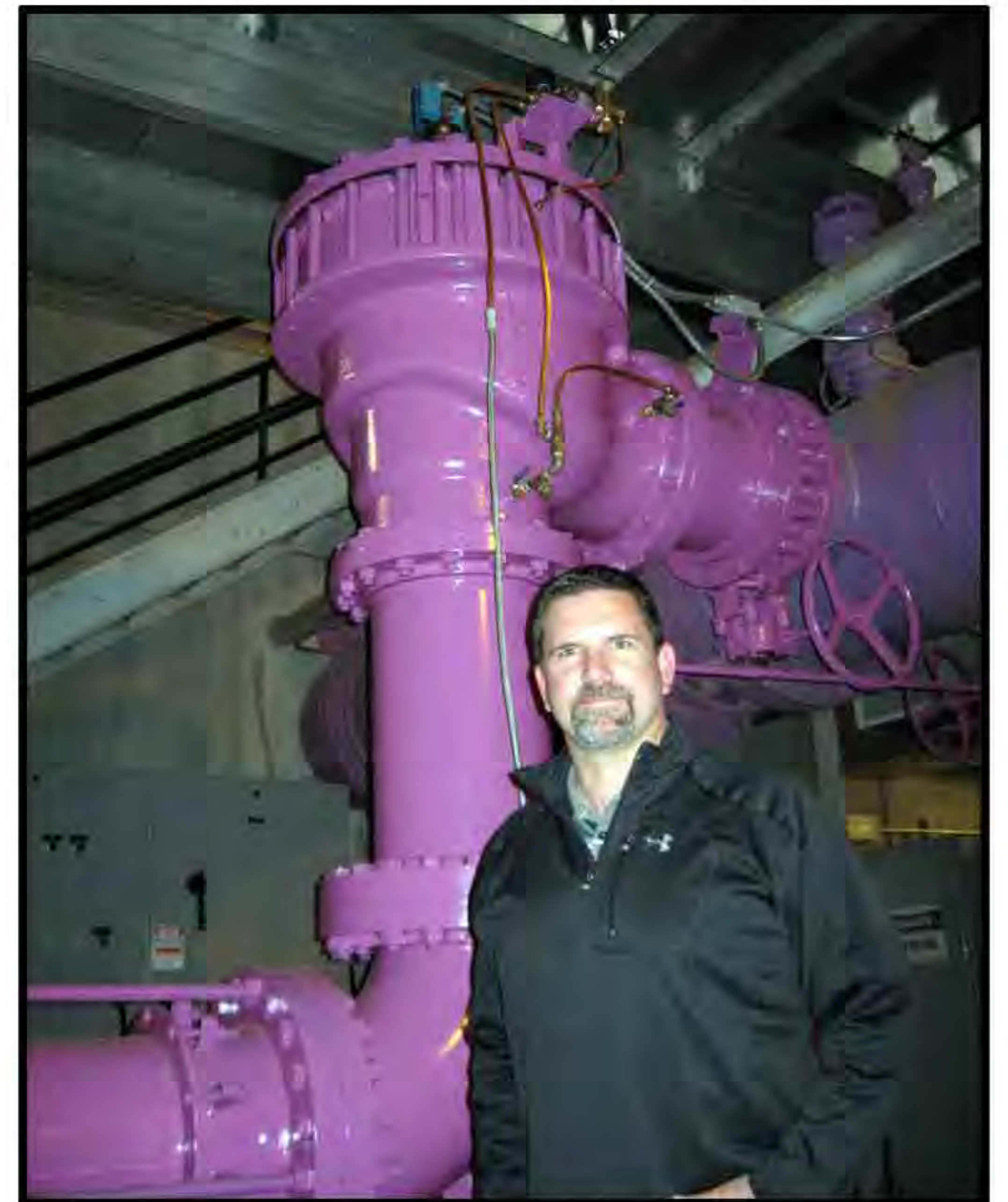
Steve at the site of the Truckee Meadows Water Reclamation Facility Pump Station retro-fit.
