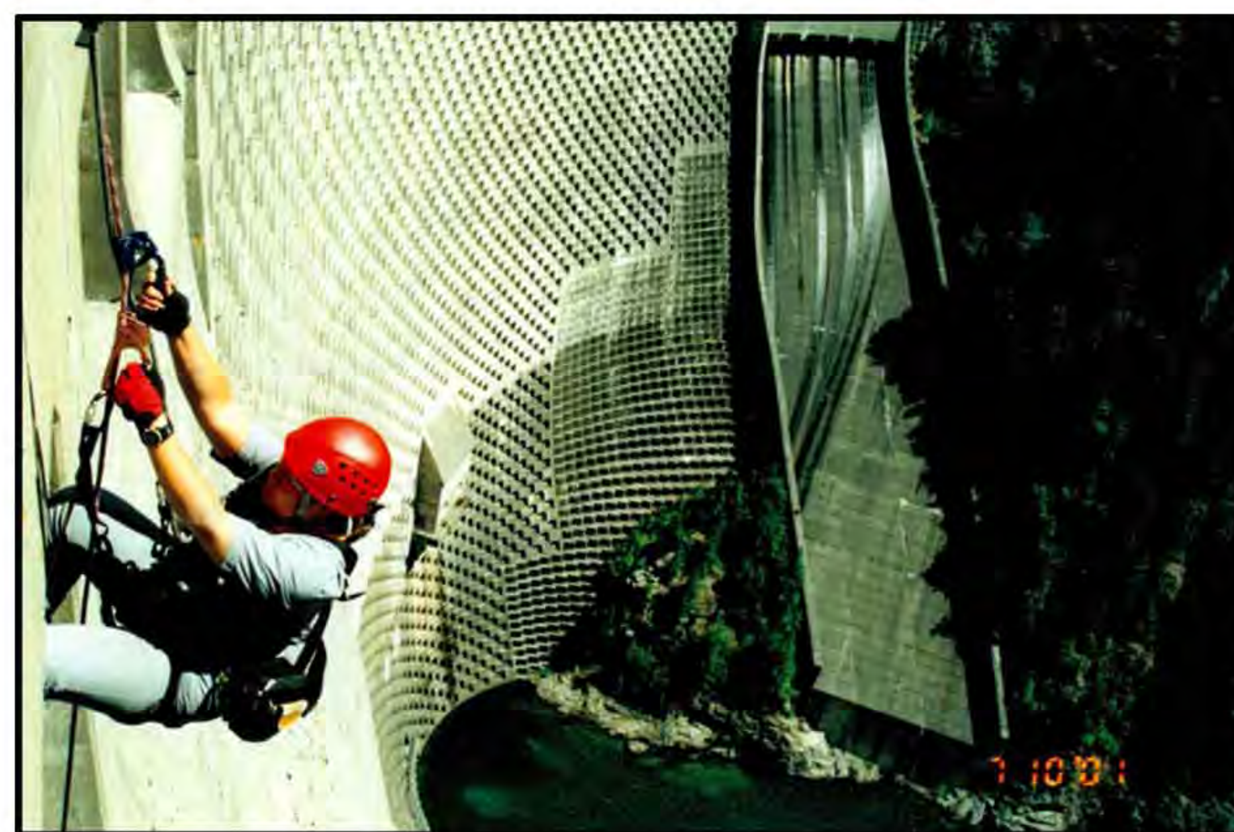
Left: Heather performing a structural inspection of Ross Dam in the Cascade Mountains in Washington State.
